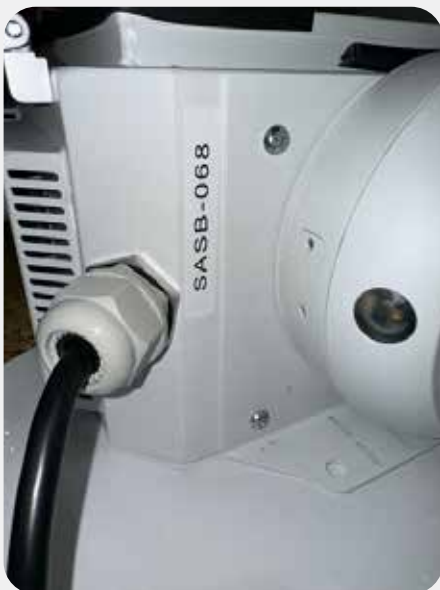
Power cords for box activation.
